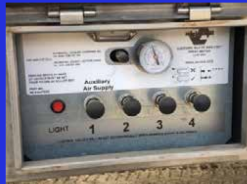
MANUAL PNEUMATIC CONTROL PANEL
